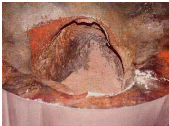
Six-inch hole eaten away by leaking boric acid from a cracked reactor drive nozzle at the Davis Besse nuclear power plant in Toledo, Ohio. Discovered and photographed in 2002 and plant shut down to avoid potential core melt down. Photograph from Nuclear Regulatory Commission .
